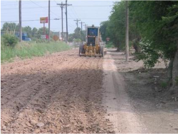
The whole of the road is prepared at the proper depth to receive the water product treatment
